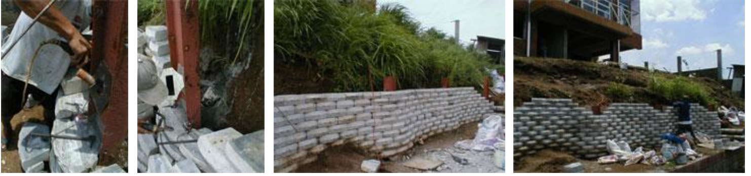
Welding of 12 mm re-bars to the I -Beams, LocBloc wall proceeds upwards until Tenth Level-wherein the same process of inserting 12 mm re-bars,grouting of 'grooved' LocBloc and welding them to I-Beams occurs again.
