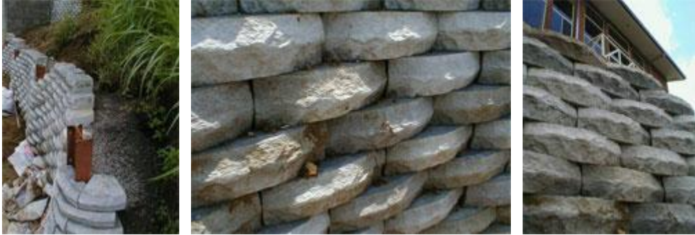
Backfilling of areas behind LocBlocs with waste sand or gravel ('gravitas'), close-up of 'built - in' weep holes of the LocBloc (gaps formed by the irregular contours of the LocBloc face ).
